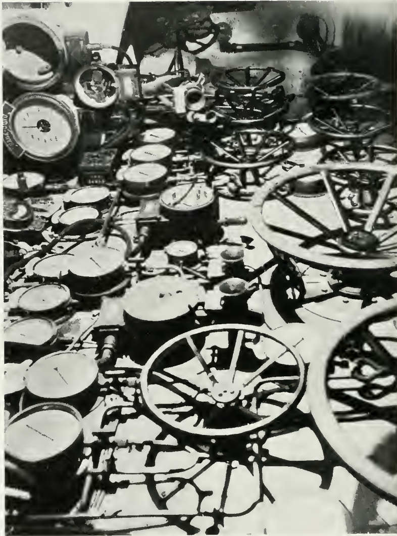
ENGINE-ROOM CONTROL BOARD, "EMDEN."
